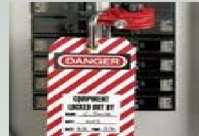
Circuit Breaker Lockout
